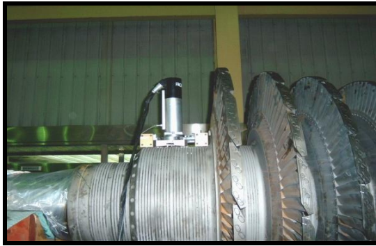
Boryeong thermoelectric power plant
