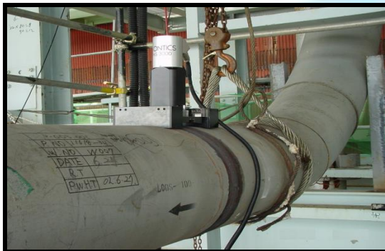
Youngheung thermoelectric power plant
